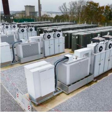
New battery energy storage facilities at Aghada Power Station
